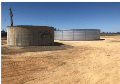
Formby South Tanks
